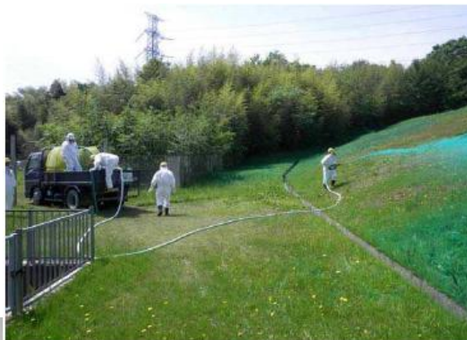
Dispersion of inhibitors in the Power Station (slope)
